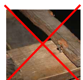
Top Edge Board Splintered
