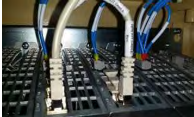
Figure 5-147: Cables at Top of Module
