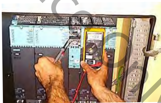
Figure 5-145: Measuring the DC Voltage
