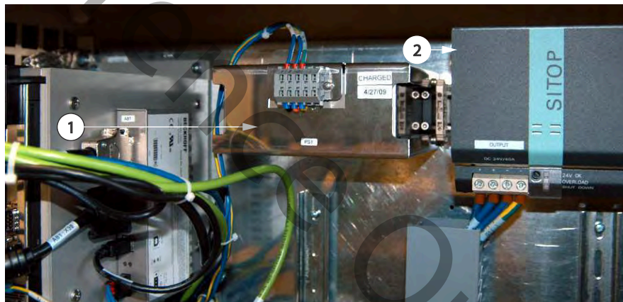
Figure 5-140: UPS and Battery (Typical)
