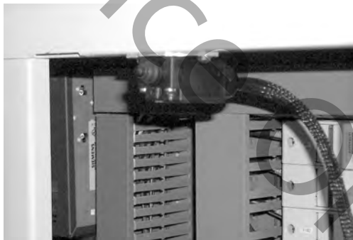
Figure 2-11: Electrical Cabinet Door Interlock Switch
