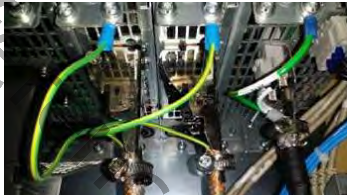
Figure 5-148: Cables at Bottom of Module
